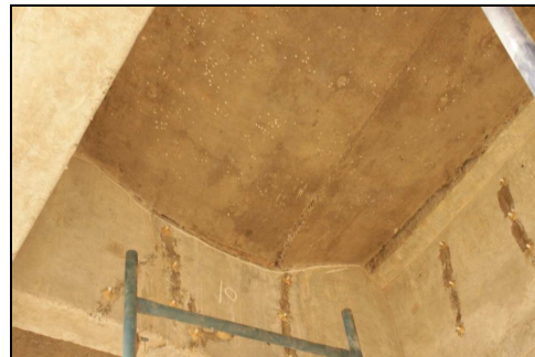
Fig.13 Distressed slab from below
