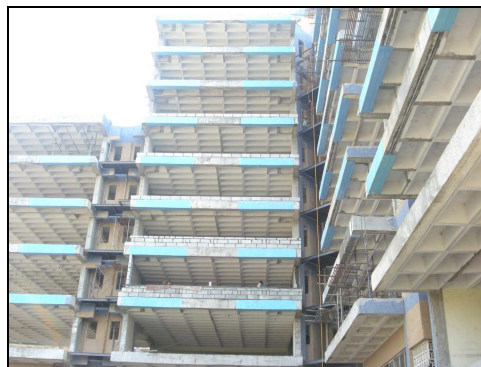
Fig.26 Final view of the building after strengthening of beams by using FRP Wrapping. It is visible on the beams as blue color.
