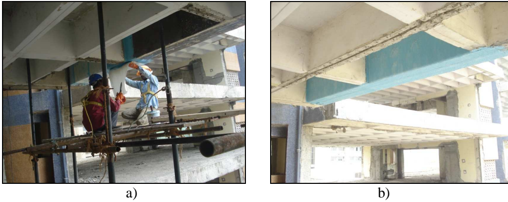
Fig.25 a) Fiber Wrapping of beams in progress b) View of beam after fiber wrapping
