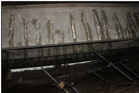
Fig.12 Cracks present on the JNPT bridge
